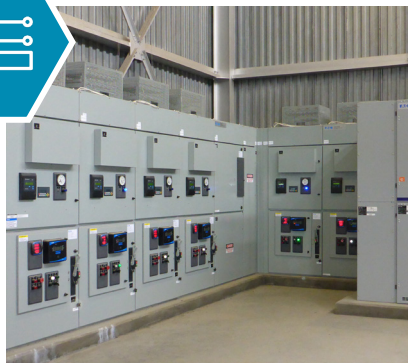
Electrical, Telemetry, Controls
